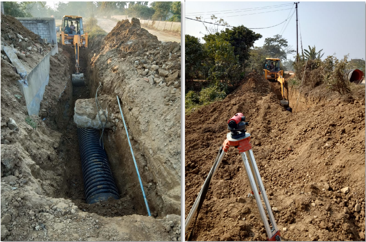
Picture 1: Installation of sewer line at Dimapur by the PHED Department for Sewage Treatment Plant (STP)
