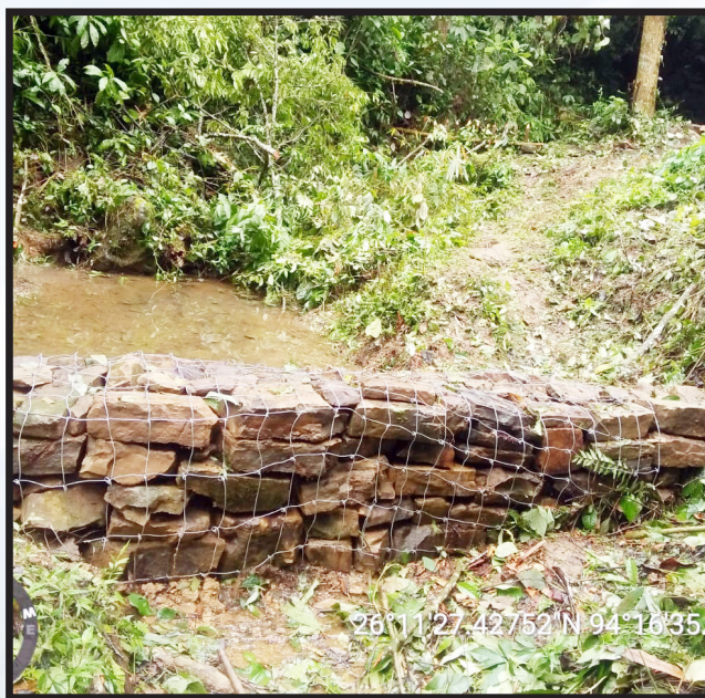
Gully plug at Rampung stream
